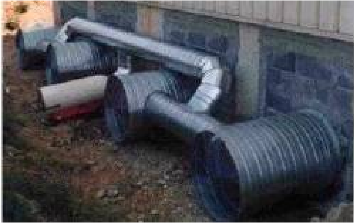
Four ventilators with one warm air generator
