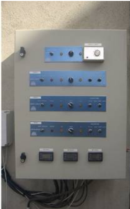
Switchboard box for three ventilators.
