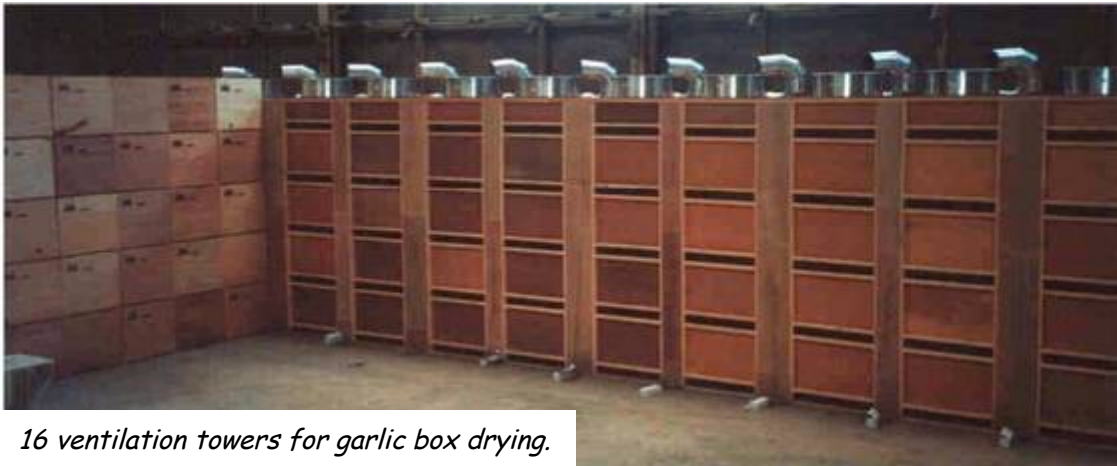
View from the back of the ventilation towers. Warm air blowers and main ambient air ventilators.
