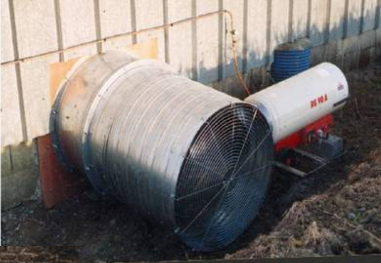
Ventilator with a warm air generator
