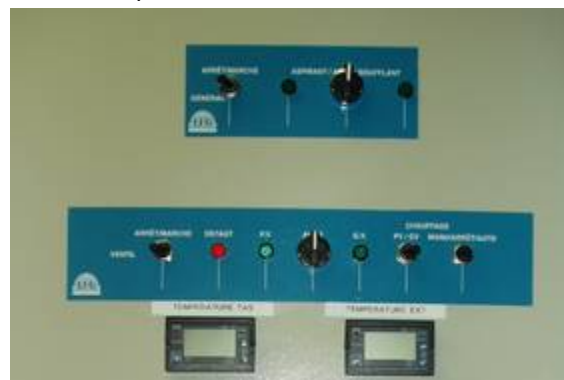
Example of automatic control system box.
