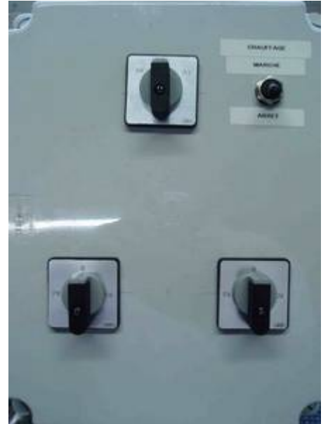
Manual order box for two ventilators.
