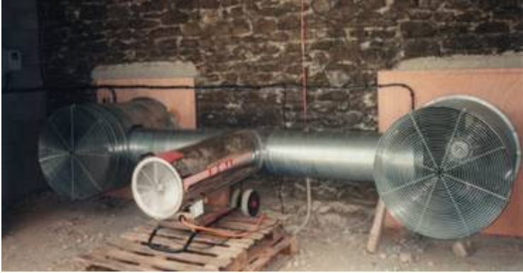
Two ventilators with one warm air generator
